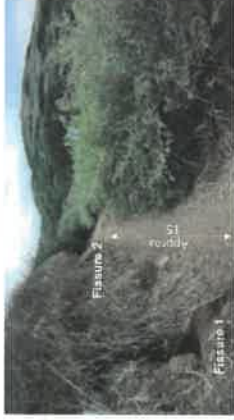
Fill Fissures Head of Klondike Slide
